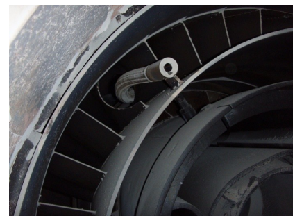
Inside boiler view of the fiber optic assembly tip
