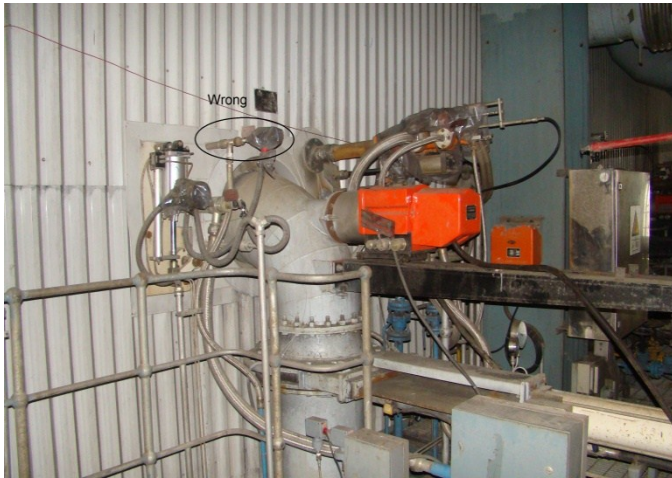
Before Safe-Fire's flame scanner modifications. The existing scanners were mounted in the wrong location.
